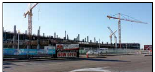
Clark Steel and Gerdau are key players in making improvements at the San Diego Airport.
